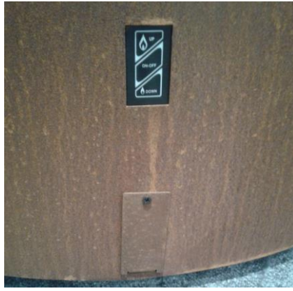
Fig 8: Receiver batteries containers
